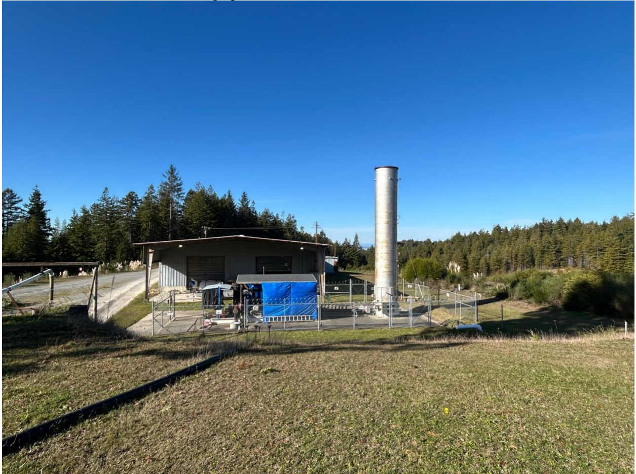
Photograph 2 –View of LFG skid and Flare Stack
