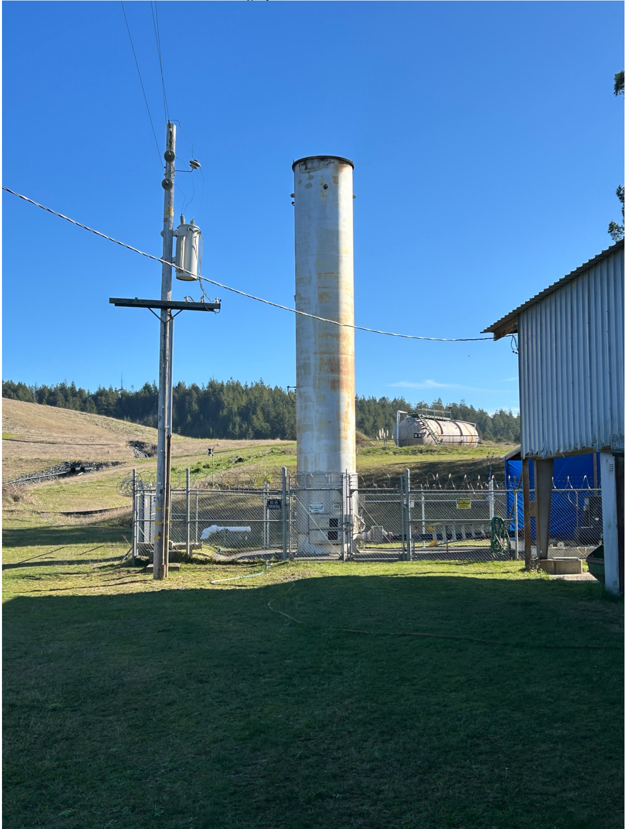
Photograph 1 – View of Flare Stack
