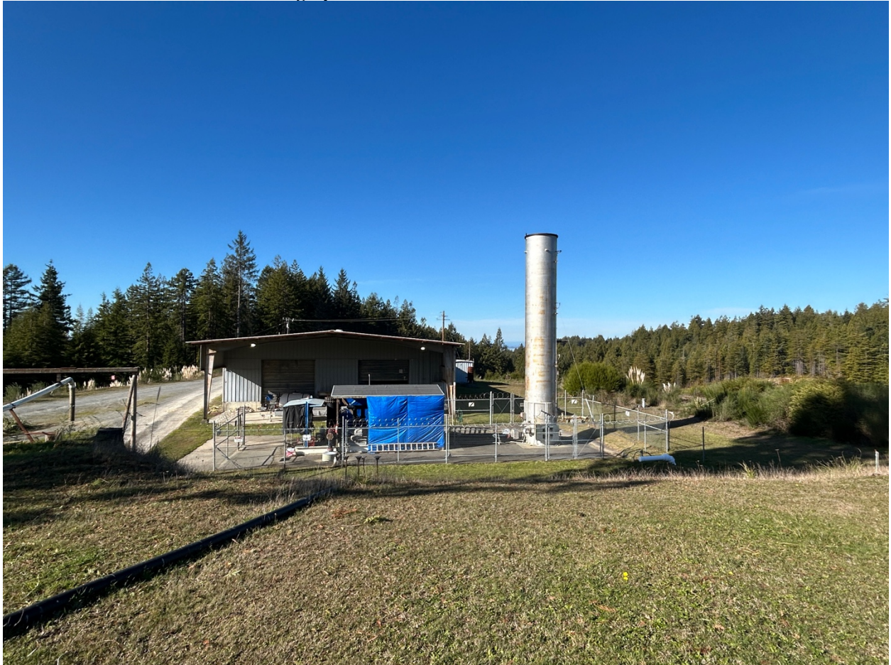
Photograph 2 –View of LFG skid and Flare Stack
